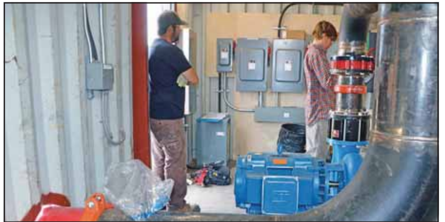
Contractors and electricians for Parkland College set up a computer software program that will operate a water distribution system at the fire training grounds east of Melville on Aug. 30. The system, which features two 100-horsepower motors, will pull water from the adjacent dugout and push it to four fire hydrants in the yard for when firefighters practise. The hydrants and underground pipes could be installed next year if funding is available. Photos by Jason G. Antonio
