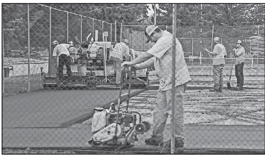
Crews were at work last week laying new asphalt on the pickleball and tennis court. The town approved $21,000 worth of work for the repairs in May. It also adopted a motion that allows any citizen who donates $150 or more toward the cost of the repairs to get a receipt for a tax deduction.
