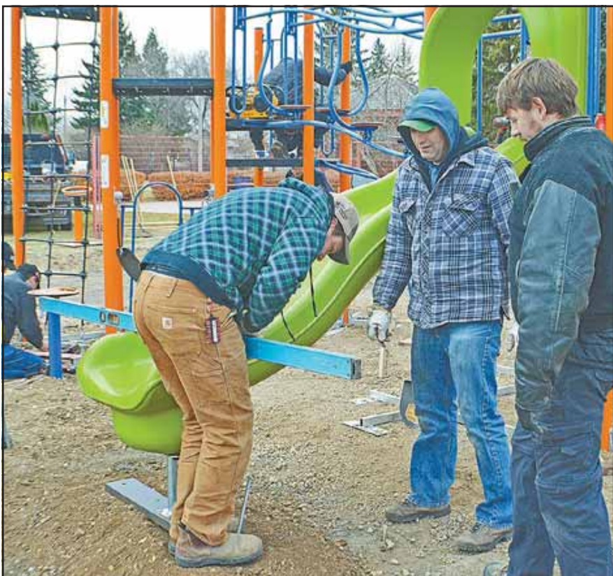
Community volunteers and workers were busy on Oct. 28, erecting new playground equipment at Kinsmen Park. The new equipment replaces older structures that were showing signs of wear.
